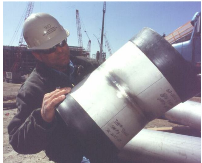
Lightweight pipe for drinking water main in sports stadium, Detroit, USA
