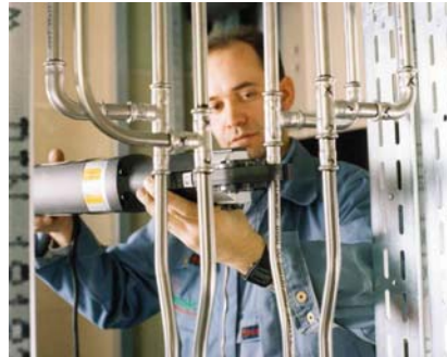
Stainless steel plumbing
